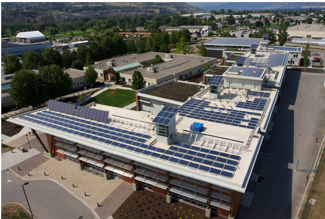
Photo: SkyFire Energy Inc
