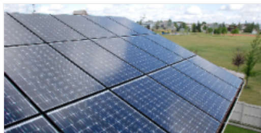
PV panels installed on a roof.
